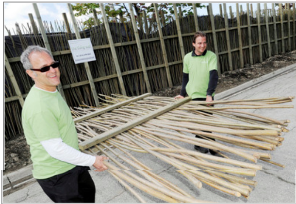
Wall of willows. Anthony Biglieri and Josef Scholbeck of The Living Wall project get dirty putting up panels of a noise attenuation barrier along Rathburn Rd. E. at Uxbridge Lane today. The wall is made of trees. Staff photo by Fred Loek
